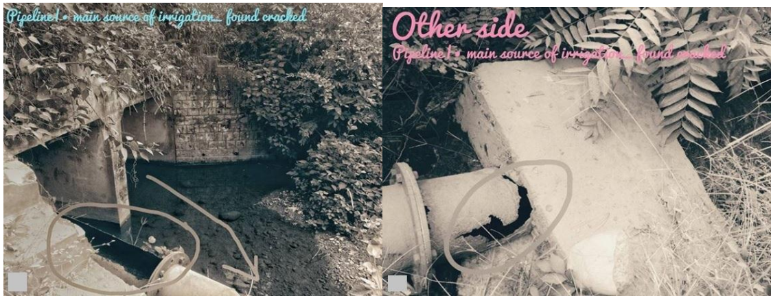
Fig (13 and 14): The steel pipe of diameter approx. 12” in the image is the main source of irrigation for the village found cracked. It is connected with a water resource from rear side and distributing the water to the fields from this starting point to end of the village via a drain which has been constructed across the village.
